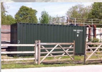
Container housing GSHP plant
