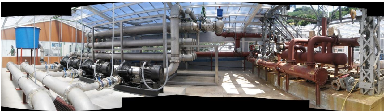
Figure 5: Heat exchanger in Barredo Shaft
