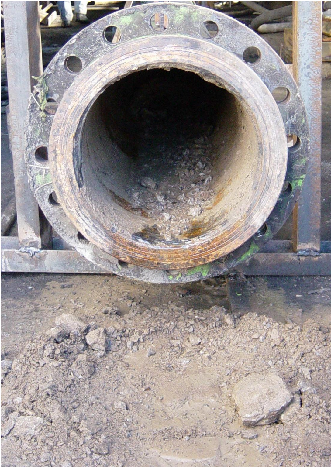
Figure 2: Depositions inside a pumping conduction
